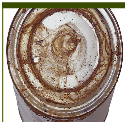
Rust that cannot be wiped off
